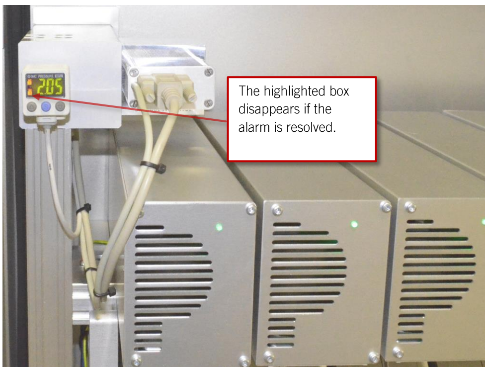
Figure 48 Cabinet inside GM12 and GM18 – Pressure indicator
